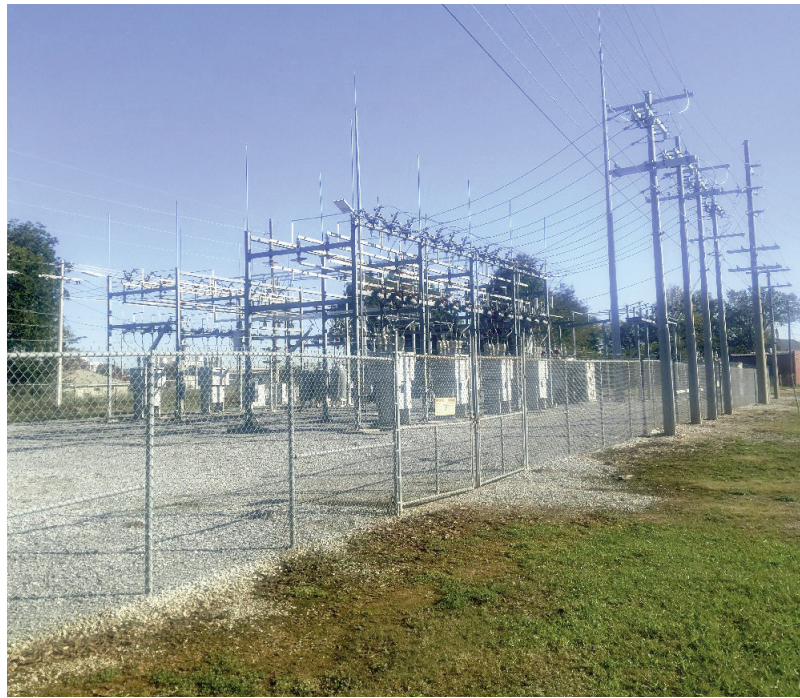
Sylacauga Utilities Board Substation #1
