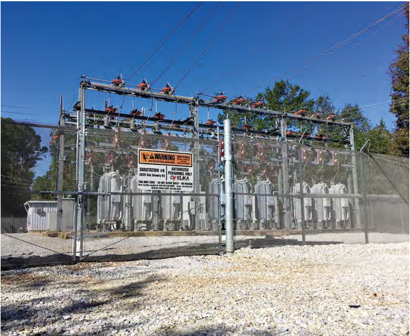
OPS Substation Number 6
