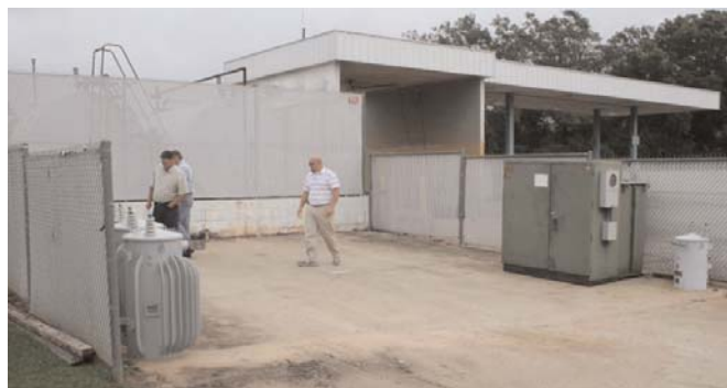
Jimmy Cluster, Fairhope Public Utilities, along with Mark Kight and Chris Phillips, Dothan Utilities, view the storage of transformers as part of Dothan's PCB Management Program. (Photo courtesy of Scott Sligh)
